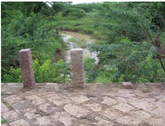
Trees and Bushes Blocked the Canal
