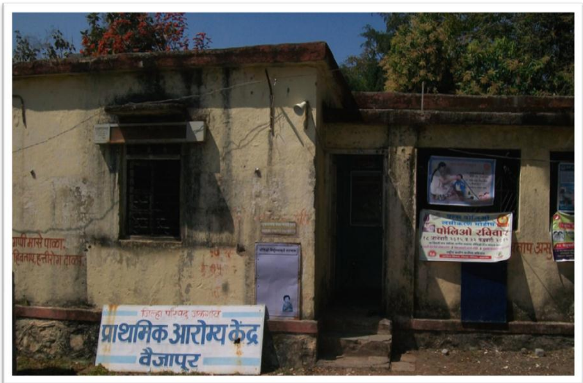
Plate No. 5 : A front view of PHC building at Vaijapur Tal. Chopda.
